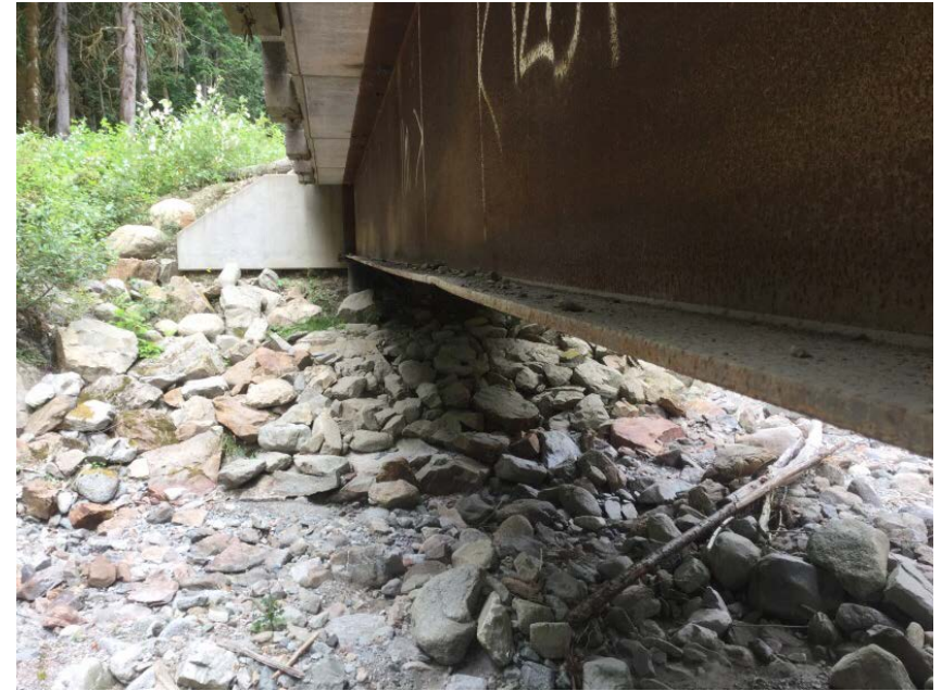
Minor damage to downstream girder, bottom flange
